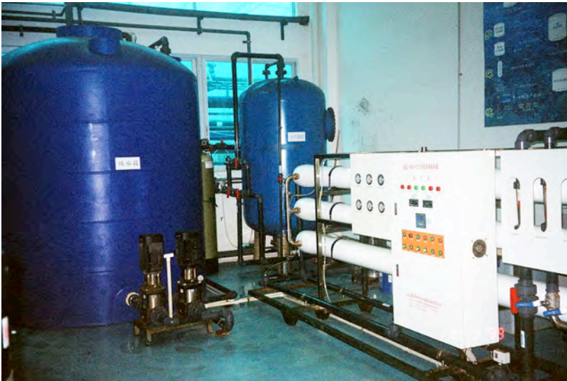
Reverse Osmosis System 55 gpm
